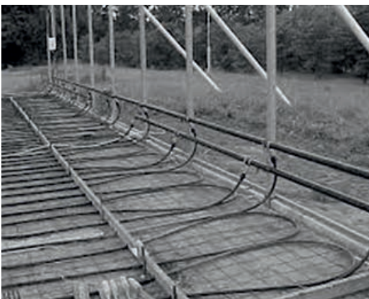
Picture 20: Ground Heating System
